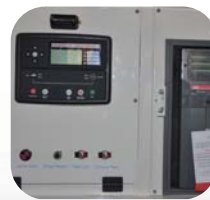
Control Panel & MCB
